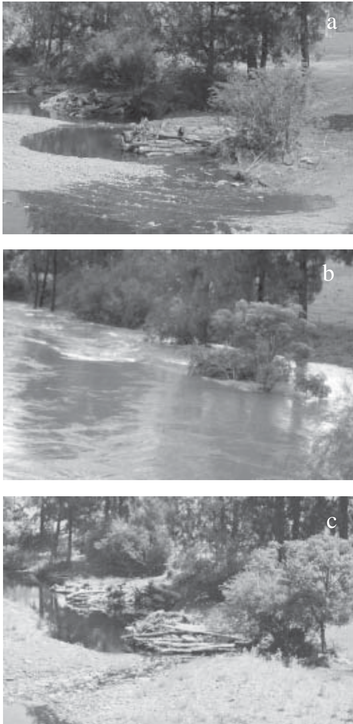
FIGURE 11. View from upstream of 2 of 15 engineered logjams constructed in the Williams River, northwest New South Wales, Australia. (a) As-built structures in September 2000, (b) March 2001 flood during which peak flow overtopped structures by approximately 2 m with velocities exceeding 3 m/s, and (c) same structures in 2002 after six overtopping flows.
