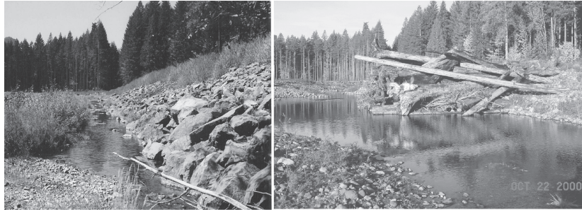
Figure 13. Photographic illustration of the differences between traditional blanket rock revetment (left) and ELJ solution (right) to protecting Forest Road 23 along Cispus River at Site B. A series of 4 ELJs was constructed to protect the road, enhance aquatic habitat, and establish a riparian buffer between the road and river. Each of the structures is approximately 7 m in height with about 4 m exposed above the low water table.
